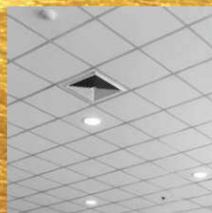
CEILING GRID FALSE CEILING
